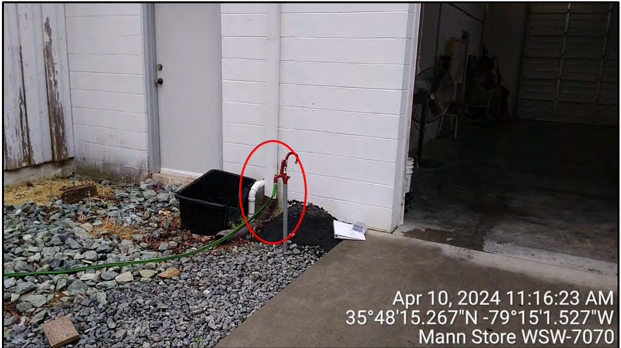
View of the spigot for WSW-7070 at the rear of the detail shop, facing southwest.
