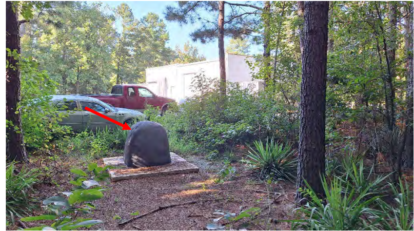
#6 – Water-Supply Well for 7070 NC 87 Site
