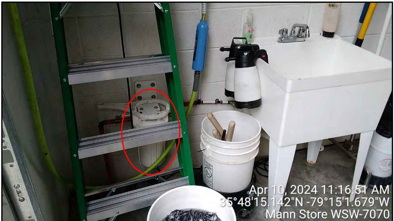
View of the filter that precedes the wash sink in the detail shop.
