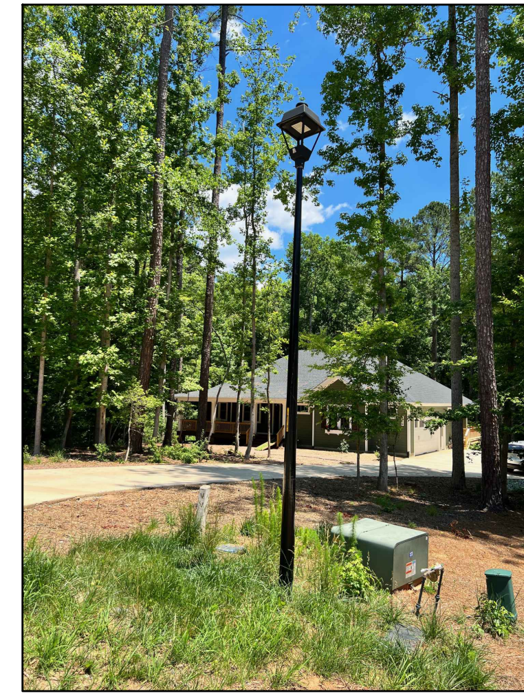
DUKE ENERGY LIGHT FIXTURES AT CUL-DE-SACS & INTERSECTION
