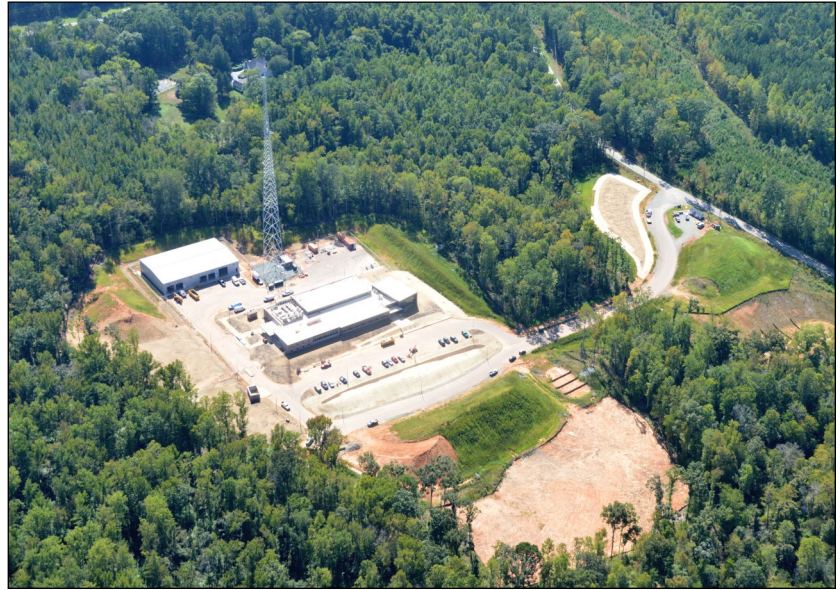
The new Emergency Operations Center and 911 Communications hub under construction on Renaissance Drive near Pittsboro.
