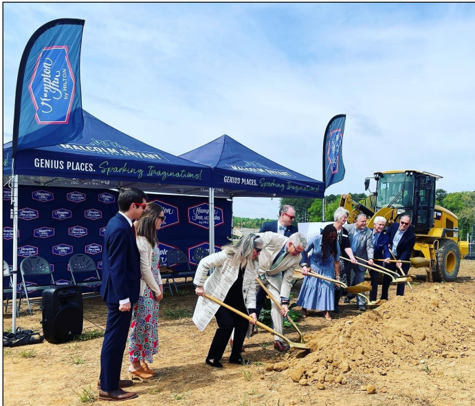
Groundbreaking of Chatham County's first hotel, Hampton Inn & Suites, Mosaic in Chatham Park
