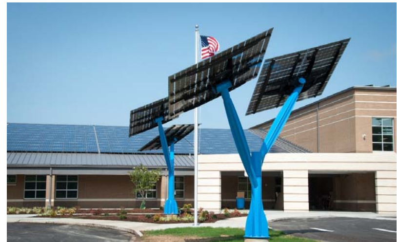
Solar trees at Sandy Grove Middle School, a net-zero school in Lumber Bridge, NC (Hoke County)
