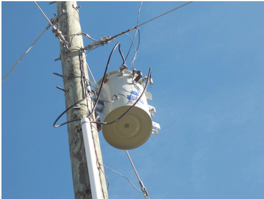
Site Photograph 13 – Pole mounted transformer (non-PCB label)
