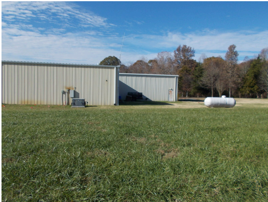
Site Photograph 11 – Propane tank and generator to west of the Property
