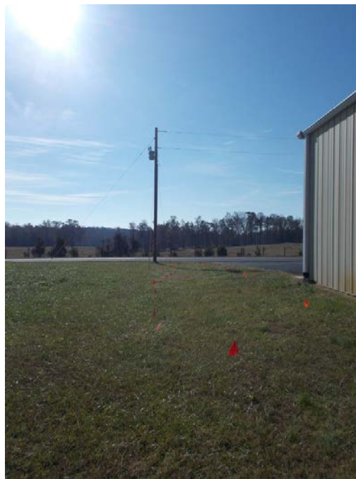
Site Photograph 12 – Pole mounted transformer and markers
