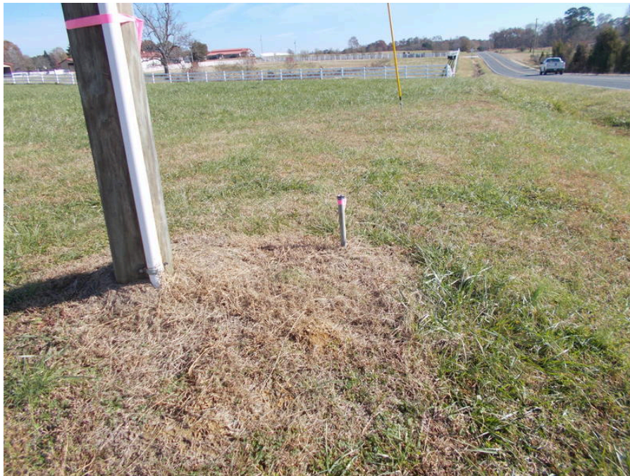
Site Photograph 14 – Metal pipe near pole mounted transformer
