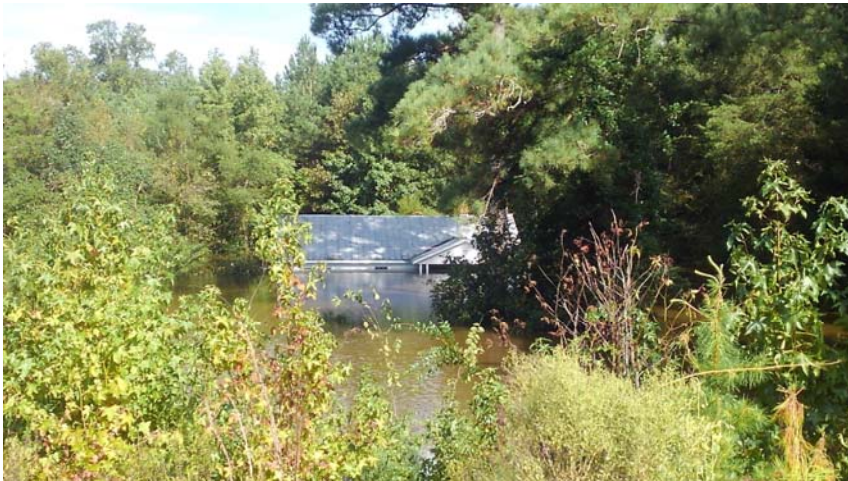
A Chatham home damaged by flooding of the Deep River
