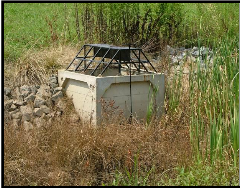
Standard Riser Outlet Small opening to dewater and larger opening at top for overflow
