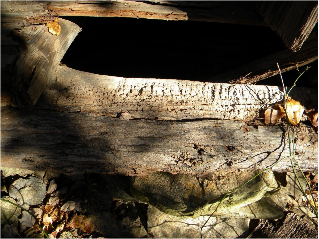
Deteriorated sill in shed addition section.
