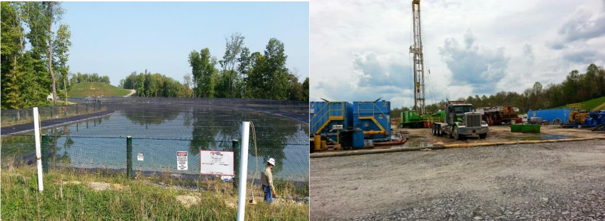
Figure 2. Typical water retention pond and well pad for fracking.
