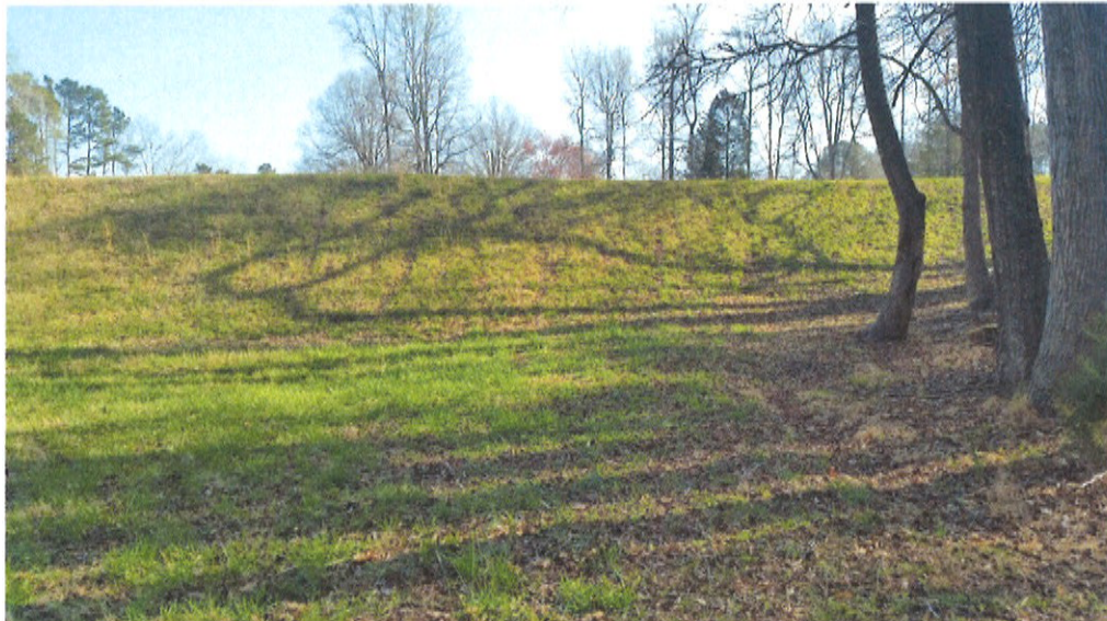
Photo 6: Below the dam of the man-made irrigation isolated pond. Up gradient view.
