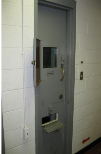
The electric controls for the cell doors must be operated at the cellblock door and cannot be used from the security of the control room.
